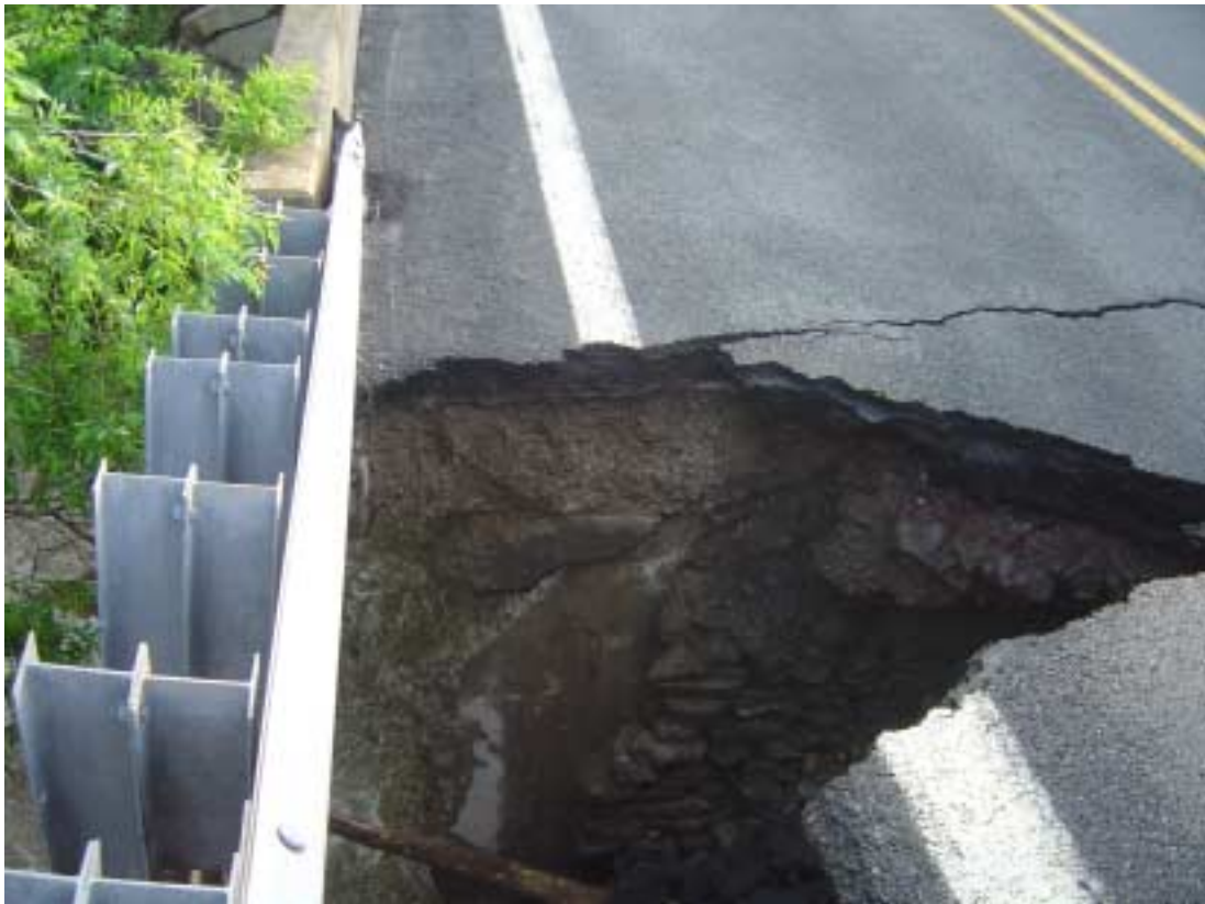
Failure at Near Left
