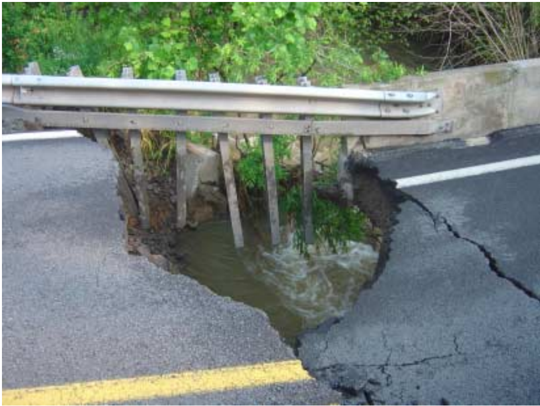
Failure at Near Left
