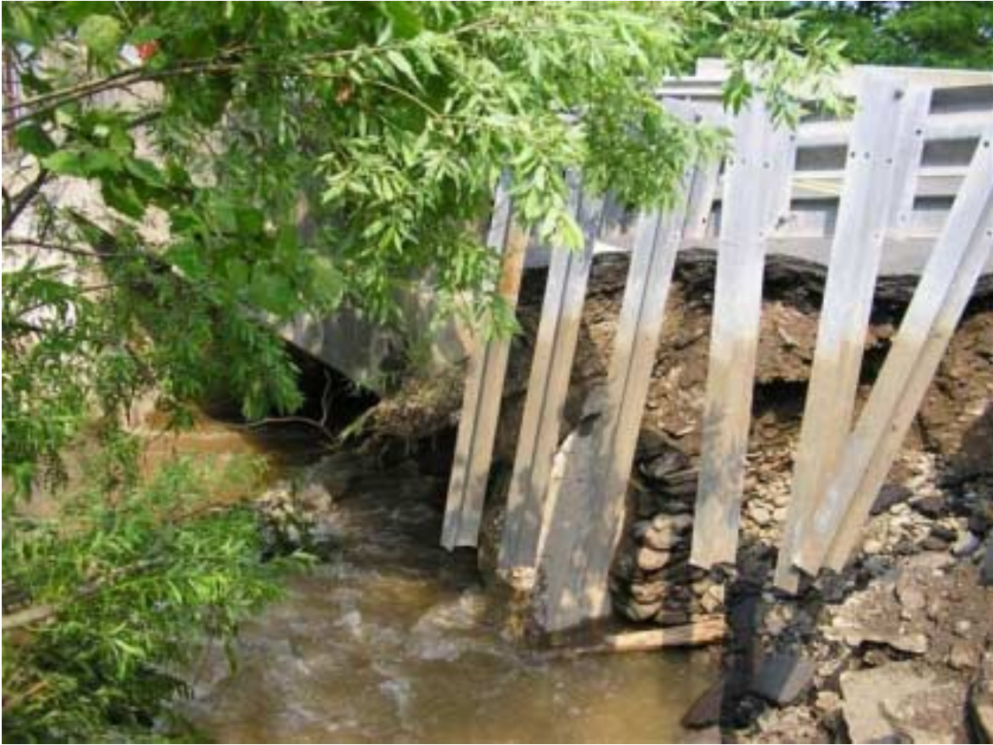
Failure at Near Left
