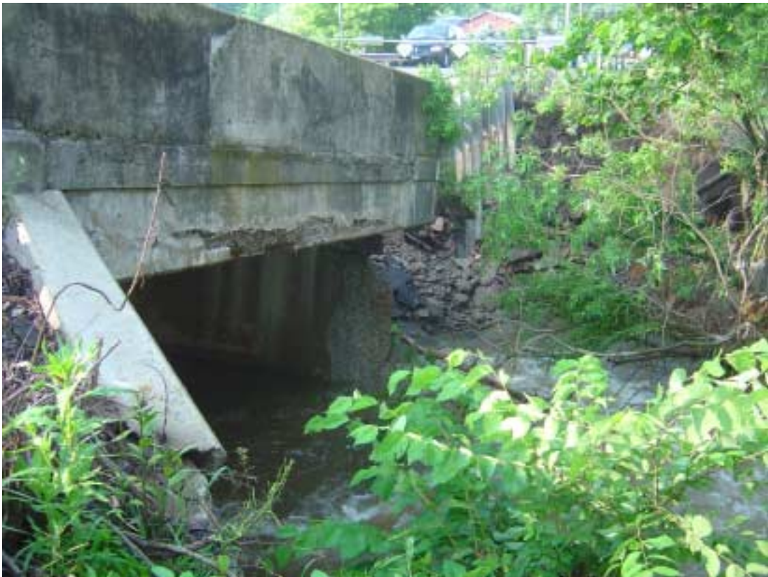
Inlet (Note missing wing)
